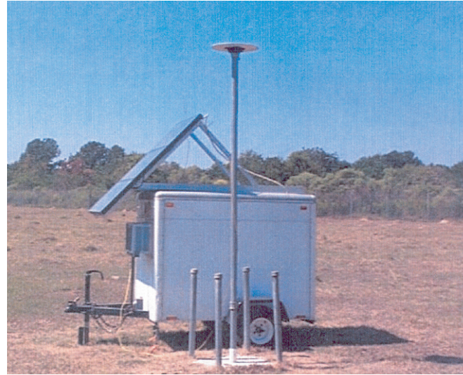
Figure 6. Trailer at PAM site.
