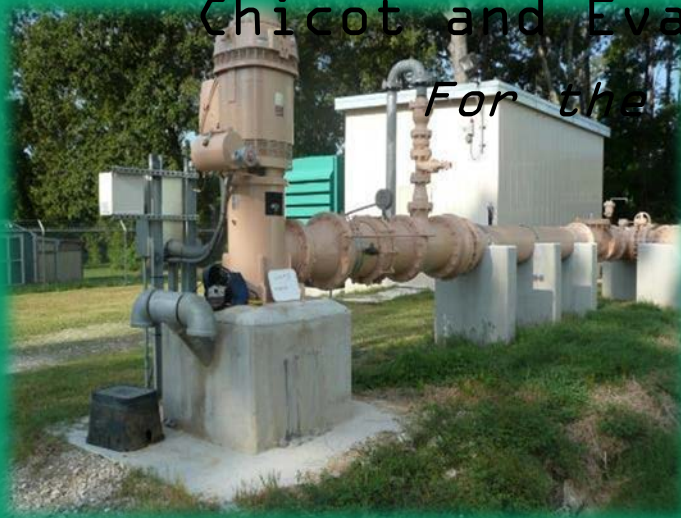
Pumping well turbine, Montgomery County, Texas
