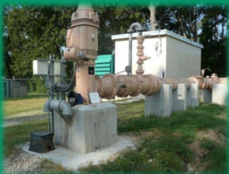
Pumping well turbine, Montgomery County, Texas
